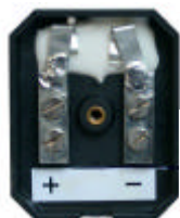
Terminal box "TB1"
