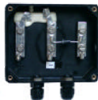
Terminal box "TB2"
